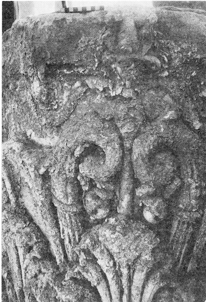
5. The salt efflorescence on the Hellenistic capitals.
