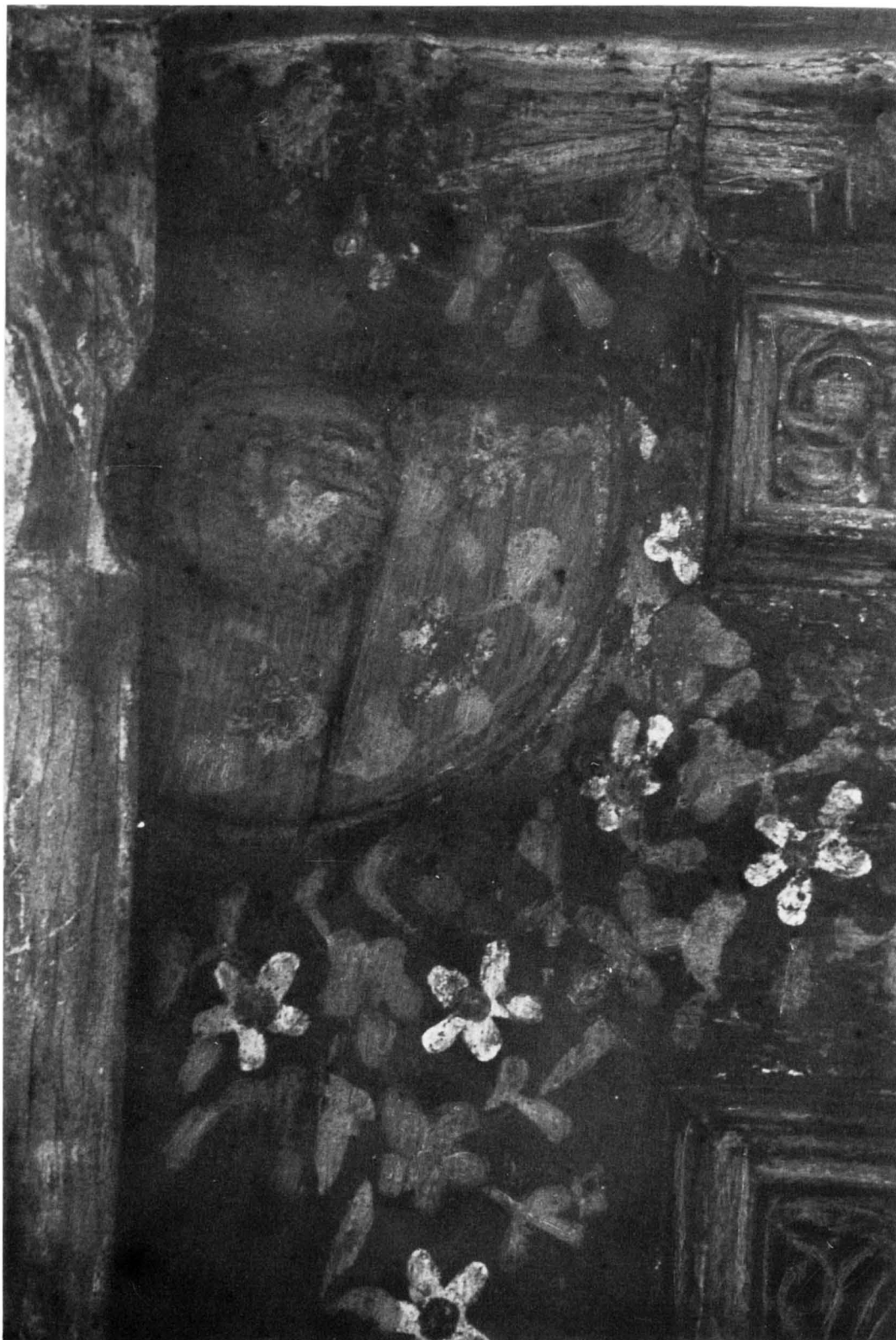
Qā'a of Ahmad Bey Kohya. Detail of soffit of the maglis showing recess for door hinge.
