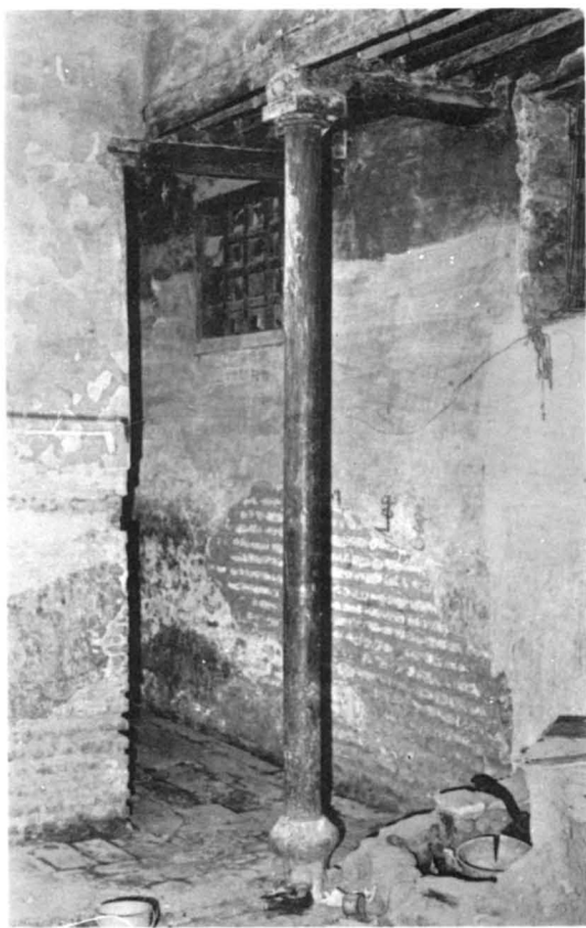
A. — First unit south staircase : wooden column near passage leading to the latrine.
